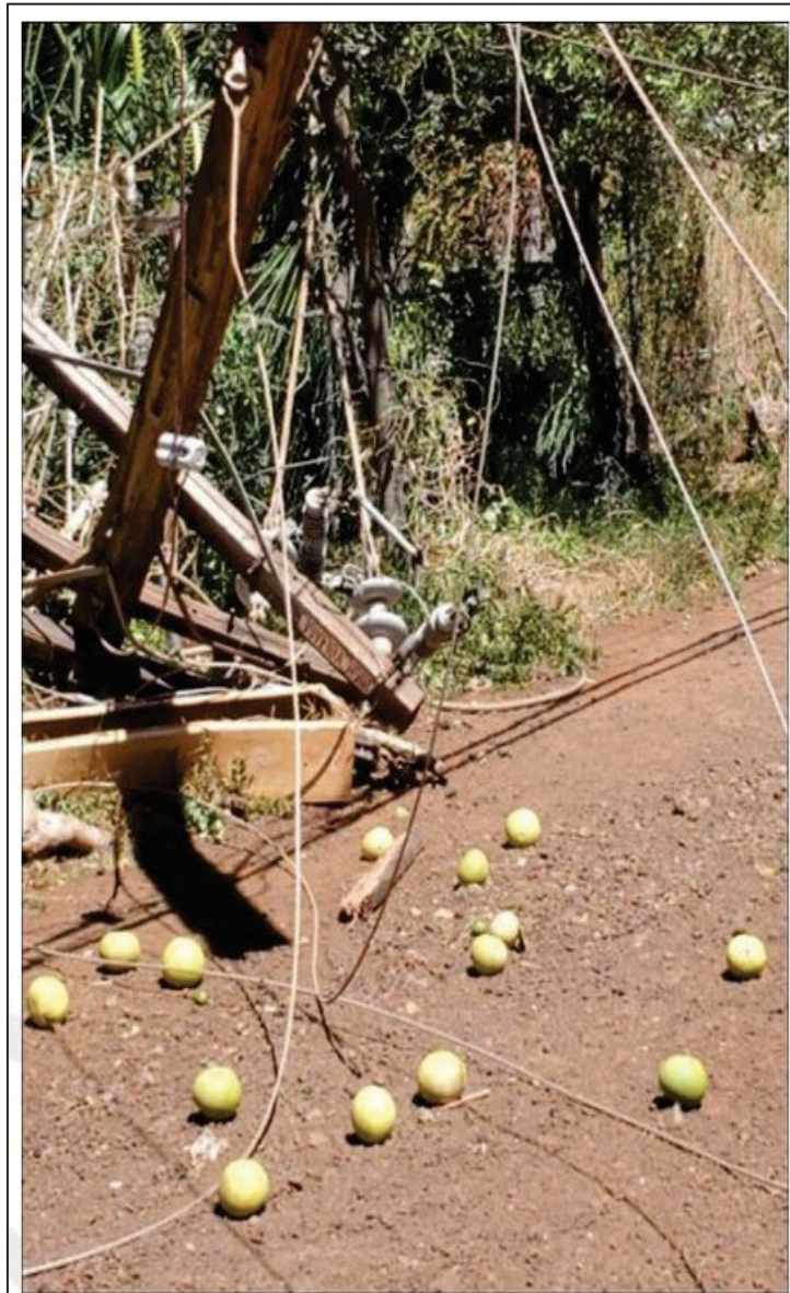
Figure 14 – Top of Utility Pole 7A on the ground
