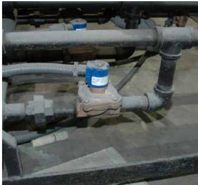
Figure 9 – Solenoid valve connected to tube bank “4”
