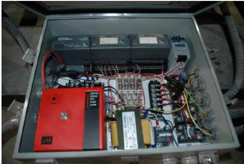
Figure 11 – Gas burner electrical circuit box containing Fireeye (bottom left corner), FieldPoint Module (top) and solid state relays (right)
