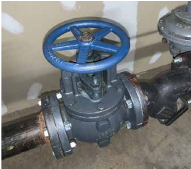
Figure 2 –Manual shutoff for Mezzanine gas train
