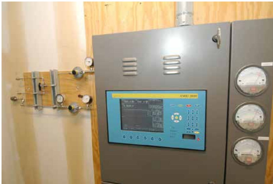
Figure 1: Combustion Calorimeter Mounted to Wall in 1 Megawatt Shed
