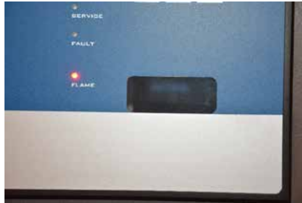
Figure 4. Pilot Flame Indicator Light and View Port.
