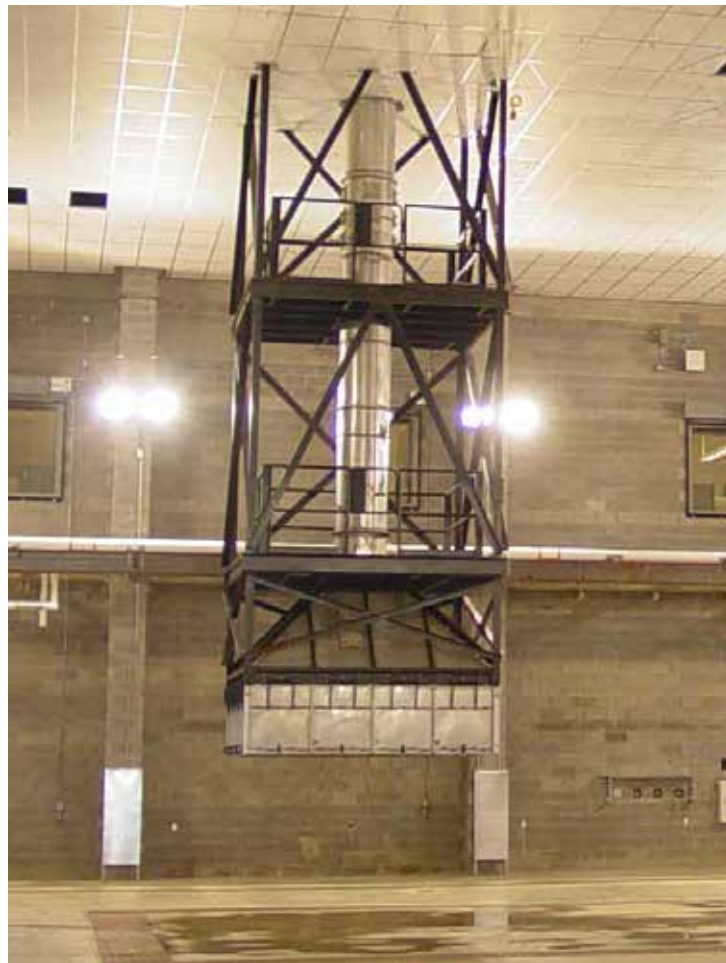
Figure 1. 1 MW Square FPC
