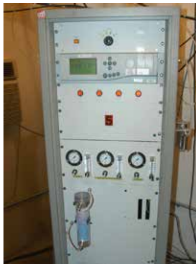
Figure 2. Rack housing of Servomex Analyzer
