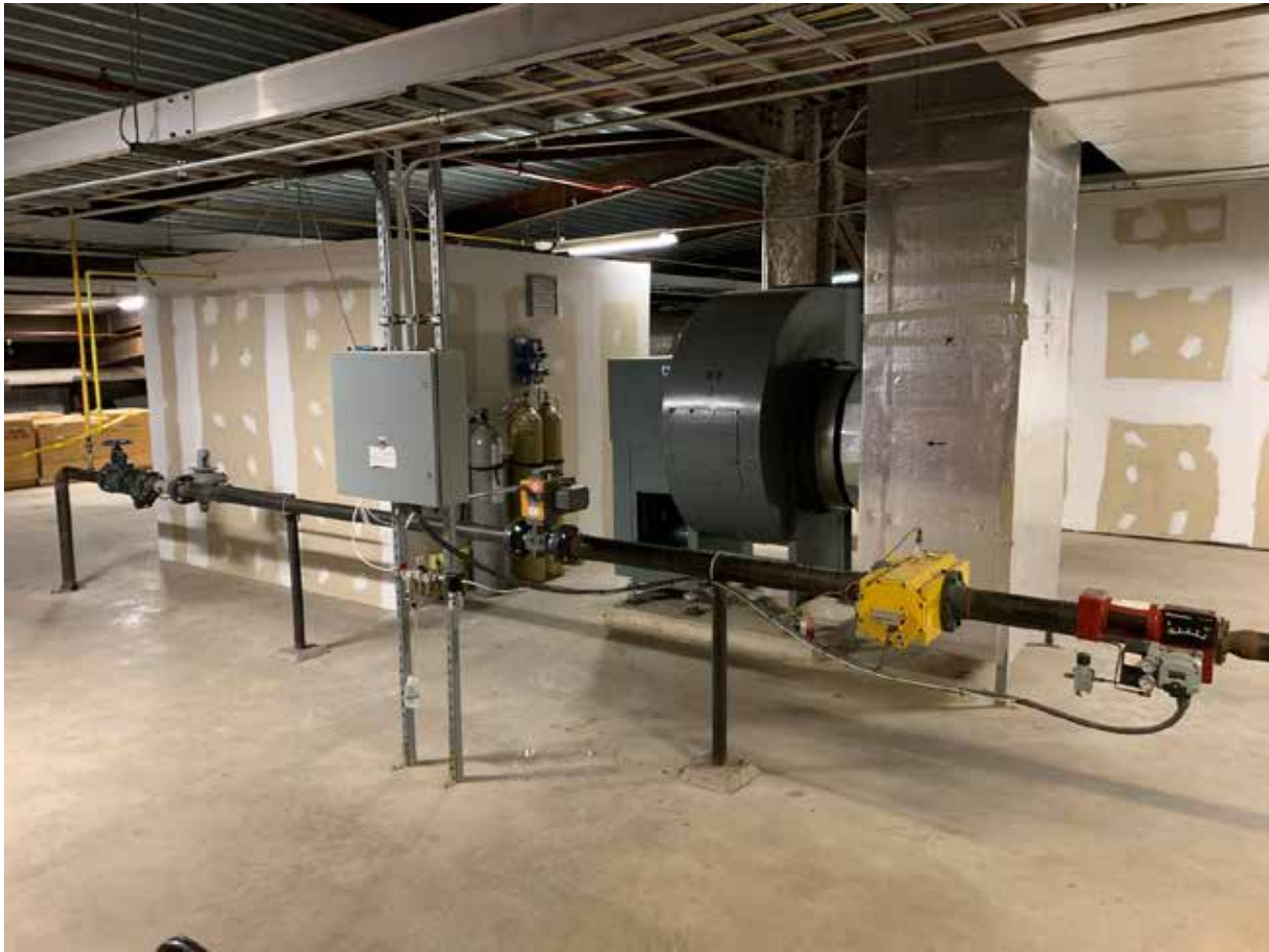
Figure 1 - Gas train in Mezzanine
