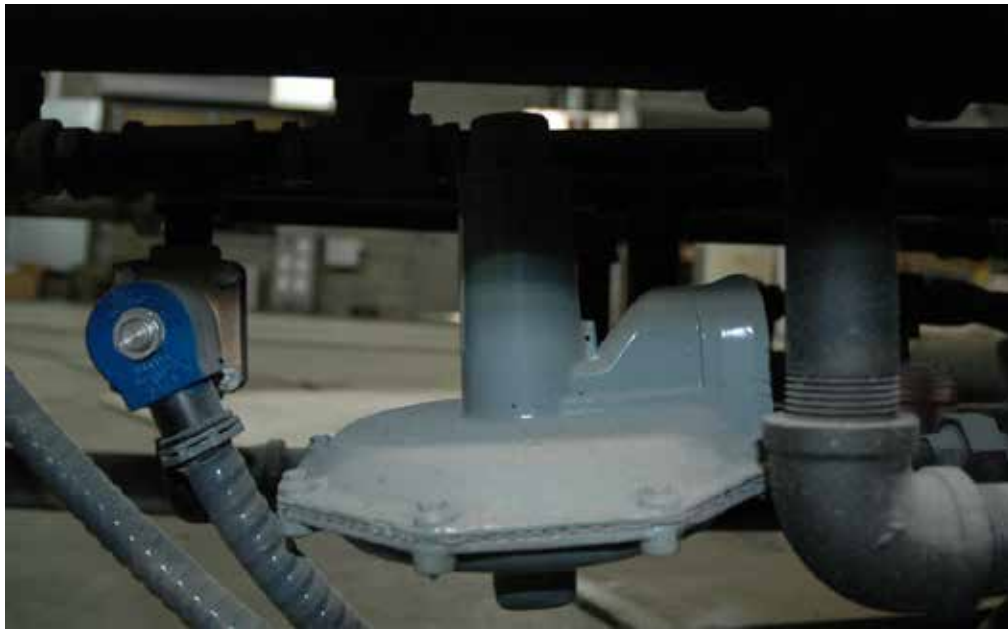
Figure 10 – Pressure regulator (center) and solenoid valve (left) for gas burner pilot tube
