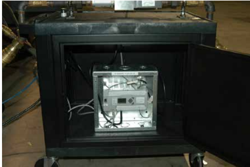
Figure 5. Allen Bradley MicroLogix 1400 PLC inside Gas Cart
